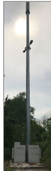
Fig. 6: End Site of BTS Hotel - Common Antenna Sharing (CAS), Power Sharing (Rectifier) and using fronthaul connectivity
